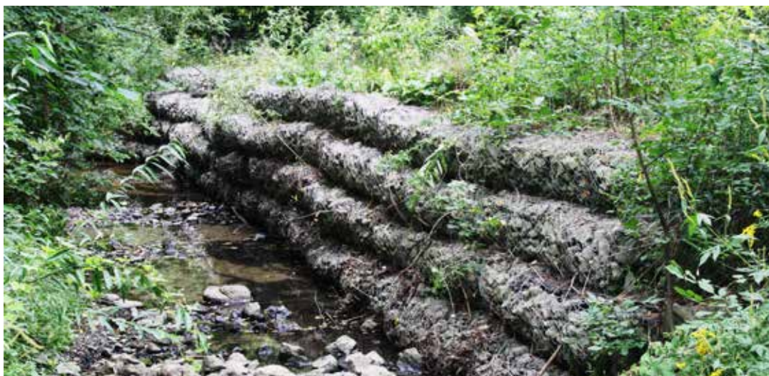
Hardened Creek Bank
