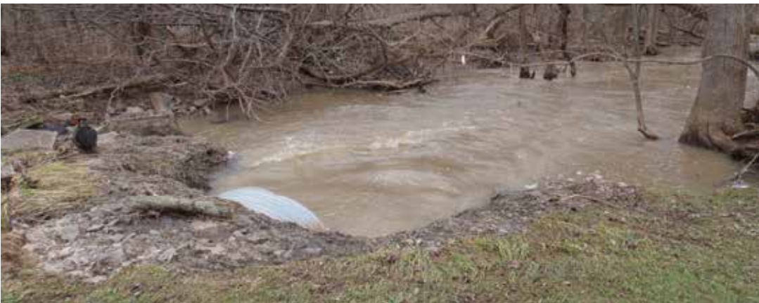
Flooding Damage - Undersized Culvert
